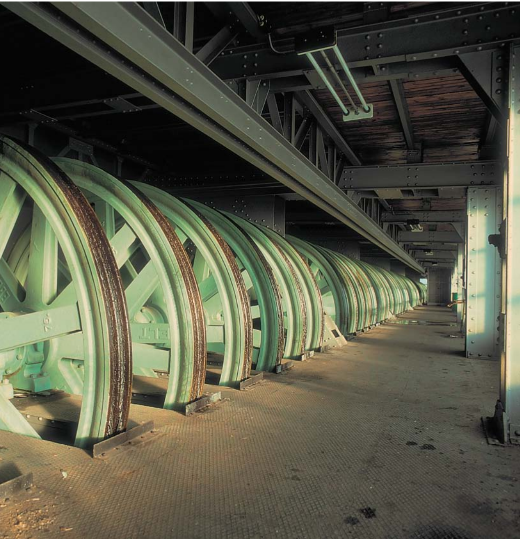
The southern line of cable sheaves on the uppermost storey of the boat lift
